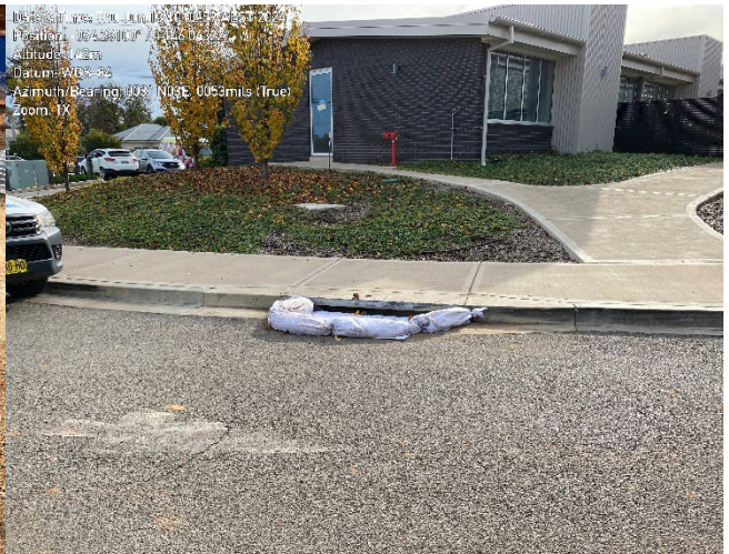
Sedimentation protection around a drain in accordance with the Project ESCP.
