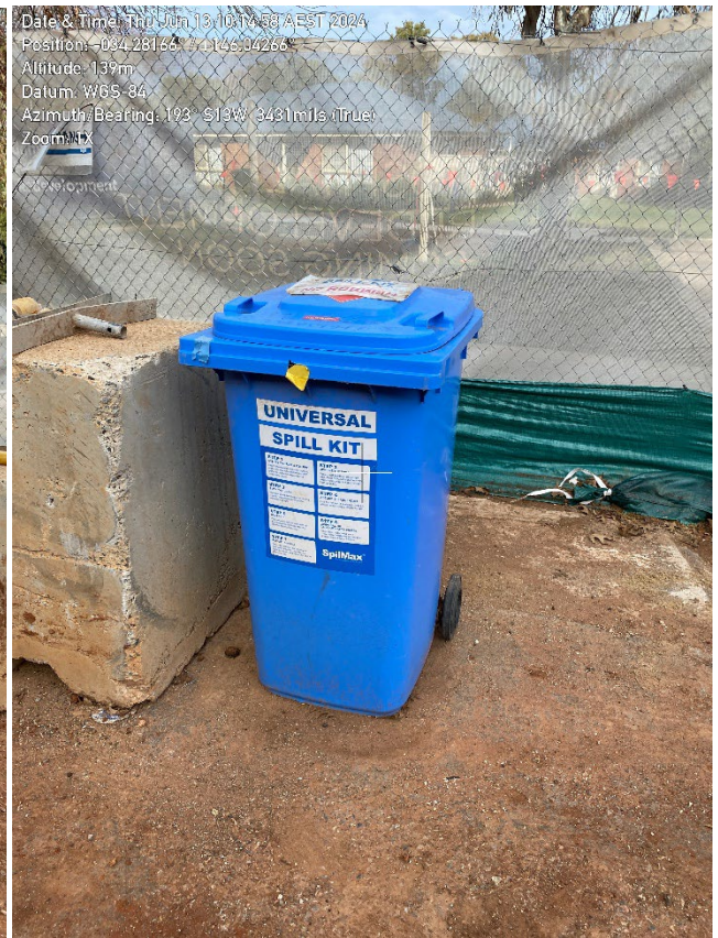
Spill kit on site adjacent to Flammable Liquids cabinet.
