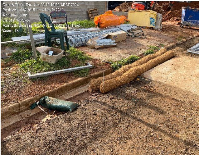
Coir logs and sandbags as sedimentation controls and stopping sediment from leaving site.
