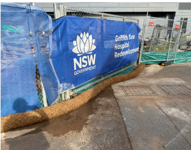
Coir logs and sediment fencing as controls along the mobile fence of the north-western boundary.
