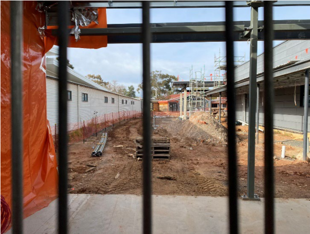
Exposed areas of soils for stormwater trenching, northern boundary, building-locked area, lower than surrounding ground-level.
