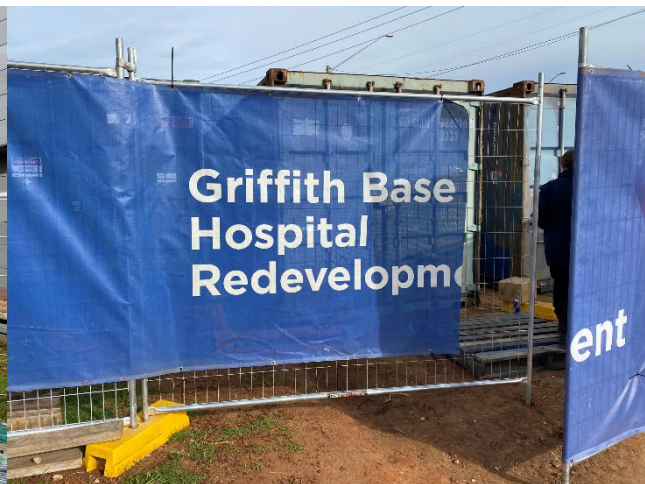
Project hoarding surrounding the site with no graffiti or third party information.
