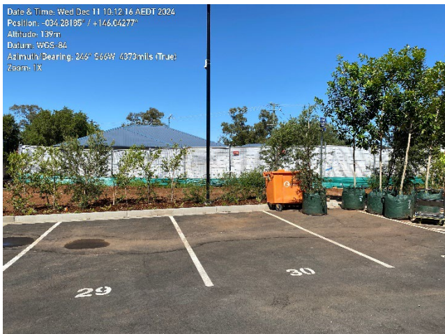
Photo 3 – waste skip, trees for landscaping and maintained sediment fence along southern boundary.
