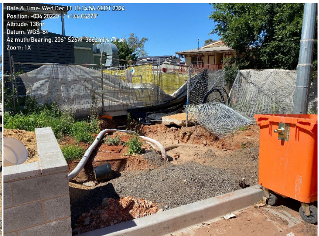
Photo 8 – area of disturbance. Trenching works occurring, lower than surrounding landscape, adjacent to eastern extent of carpark.
