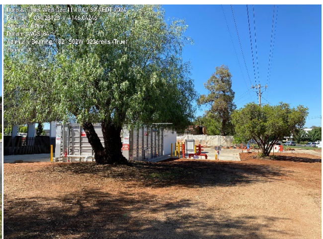
Photo 10 – tree protection has been removed.
