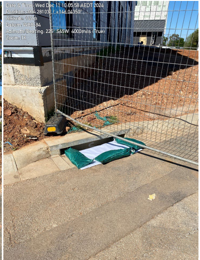
Photo 14 – geotextile and sandbags over drain as sediment control adjacent to area to be landscaped.
