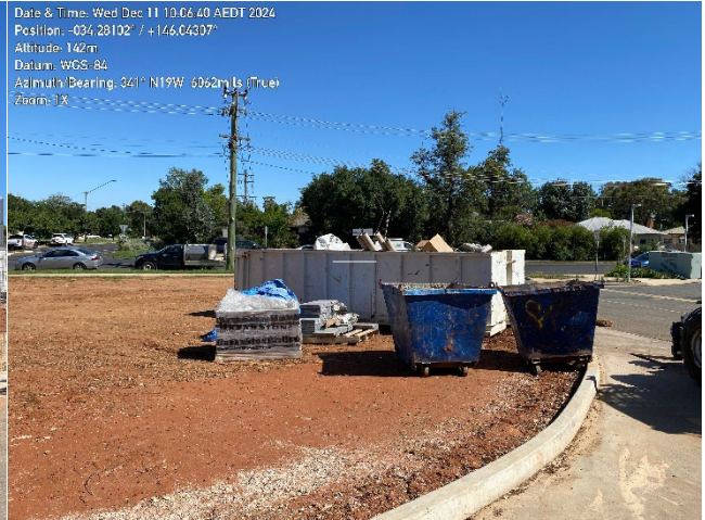
Photo 6 – waste skips in area that will be topsoiled and seeded. Site fencing and site office relocated.
