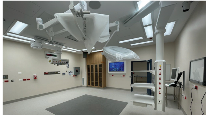
The new hospital includes two digital operating theatres, one procedure room and an expanded day surgery
